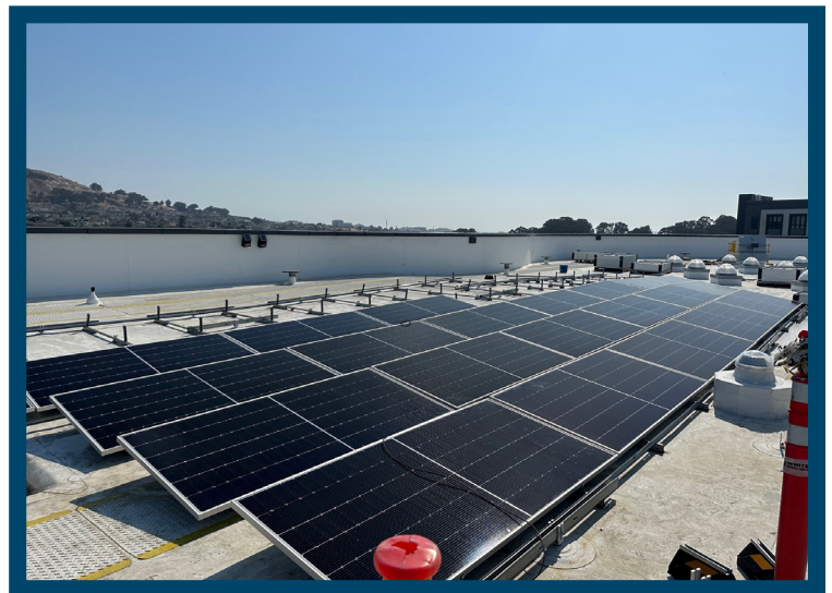
New photovoltaic solar panels at the South San Francisco Library
