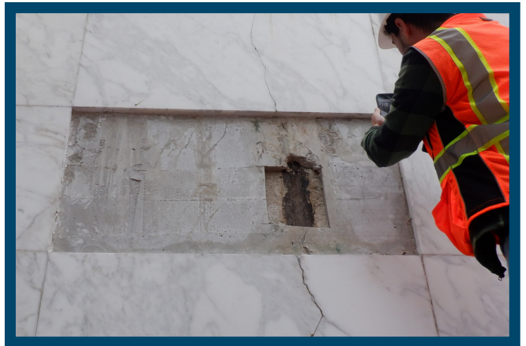
Inspecting level of damage to the facade at Santa Ana's Main Library
